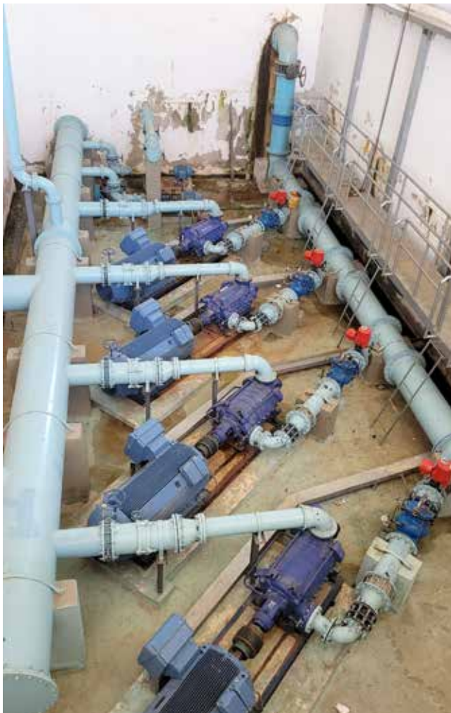
Bild: Pumpstation in Puerto Casado
